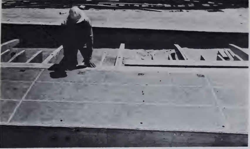
Figure 201. —Vacuum panels being constructed at Angostura Dam, in South Dakota. View shows rubber strips and hardware cloth before covering with muslin. PX-D-33514.
